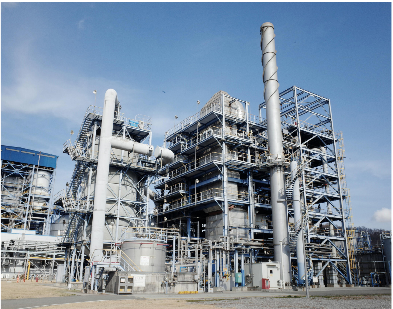
Incinerator at BASF's production site in Yeosu
